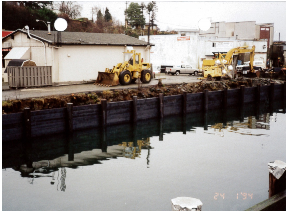
File Photos of South Section Piling adjacent to Lot 811 Harbour View Esso:
