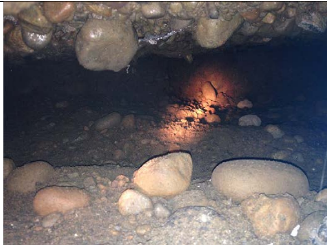
Photo #13: Testing Location #3 Northern extent of void visible in photo
