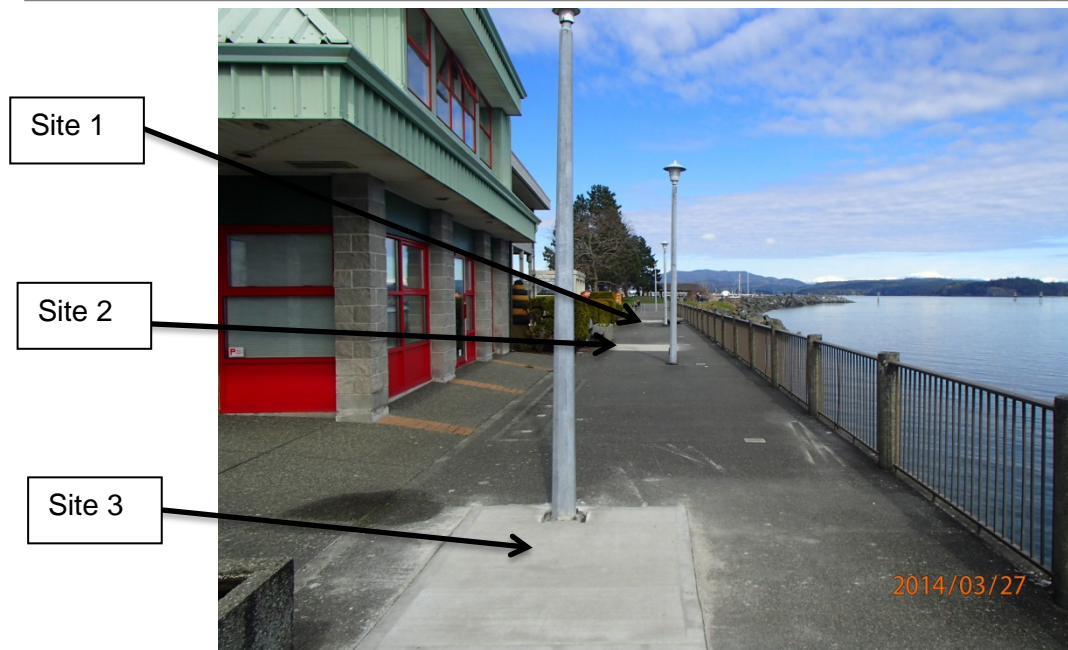
Figure 1: Location of three sites chosen for destruction. Note that all three sites are repaired with concrete and the surface of the concrete repairs is brushed.
