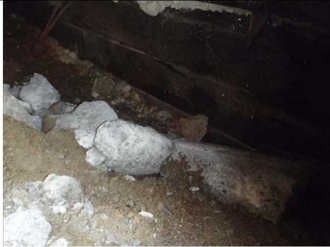
Photo #9: Testing Location #2 Void at face
