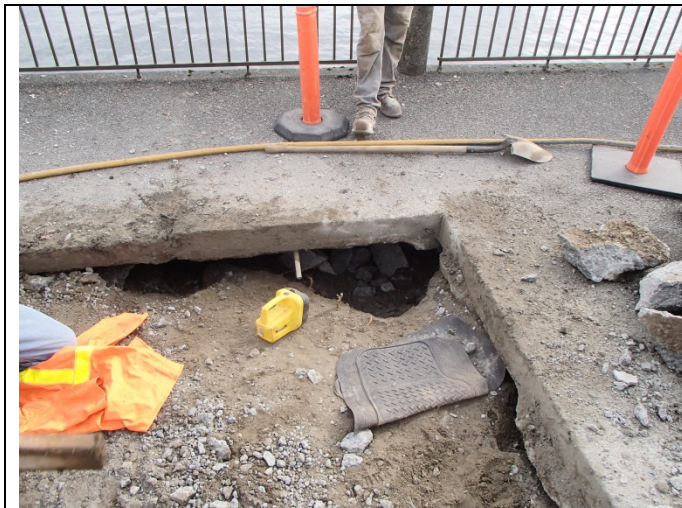
Photo #3: Testing Location #1 Fill erosion at the testing site
