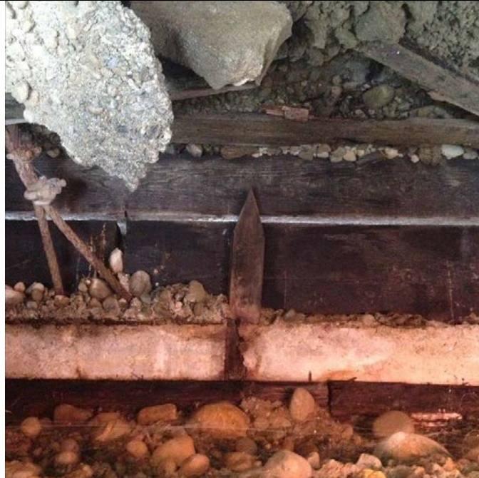
Photo #12: Testing Location #3 Void at face
