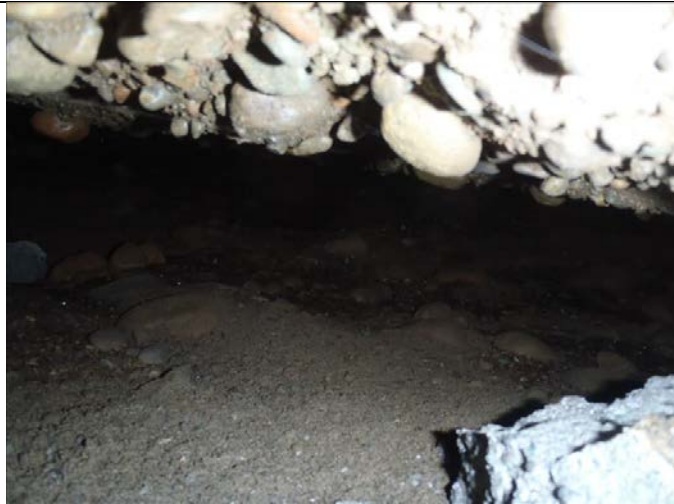
Photo #10: Testing Location #2 Looking south of testing location – completely suspended concrete cap panel
